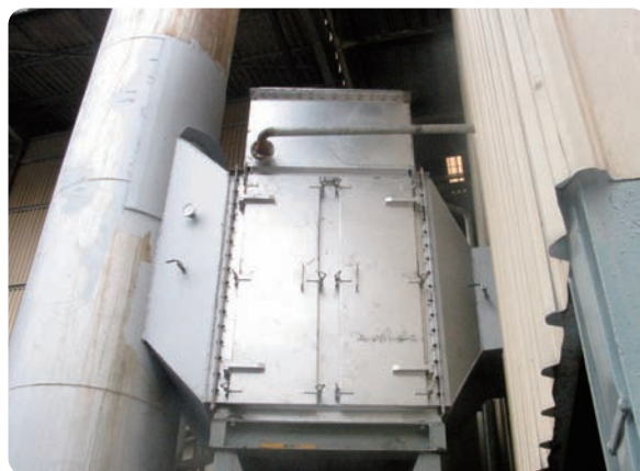
The waste heat recovery system (above) saves energy and money
